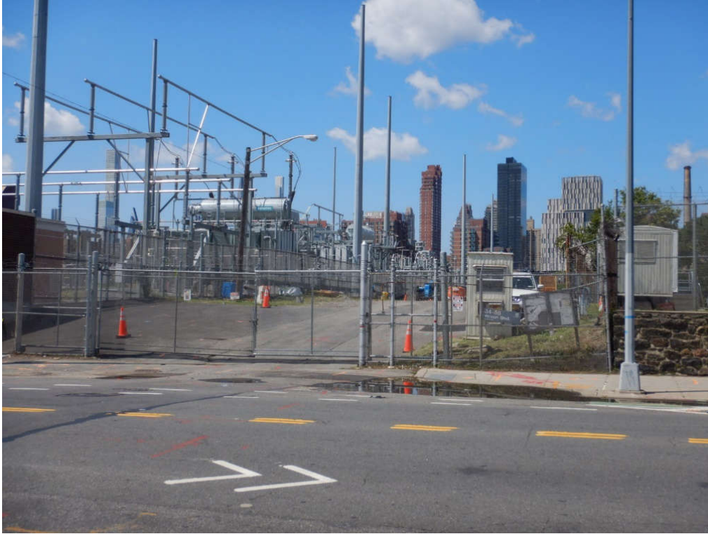
Figure 3. Rainey substation's entrance from Vernon Boulevard. The East River lies behind the electrical facility, separating Queens from Roosevelt and Manhattan islands. View facing west.
