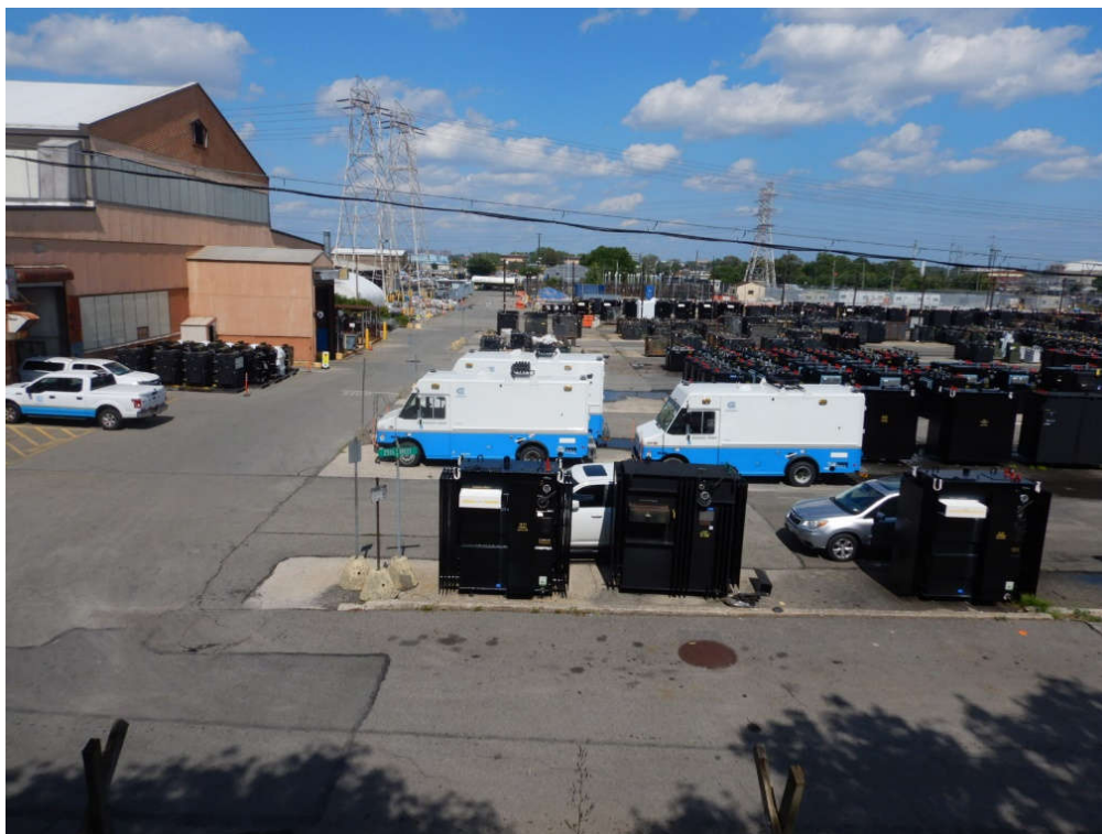
Figure 11. Astoria Annex substation area. View facing northeast from 20 th Avenue, near the Crescent Street intersection.
