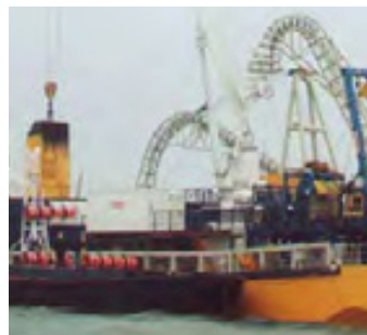
1. Early morning SeaSerpent equipment load-out on to CLV SEA SPIDER off Cowes, Isle of Wight.
