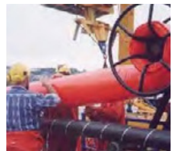
2. SeaSerpent being attached to the HVAC cable showing Seaflex manual brake RDS.
